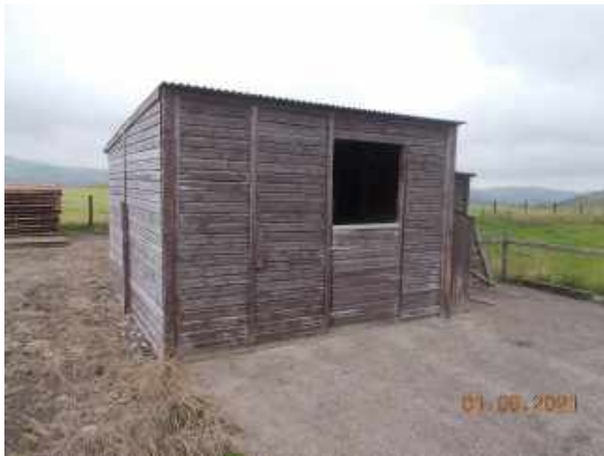
Plate 7 the small stable on the site, which will be demolished. This building was judged to have negligible potential to support roosting bats. Photograph taken from the east.
